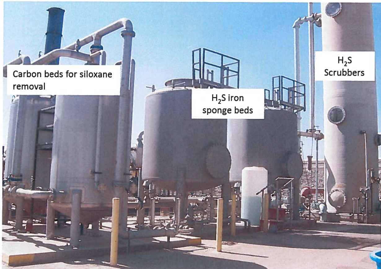
Figure F- 2 Existing Domestic Biogas Cleanup Skid
