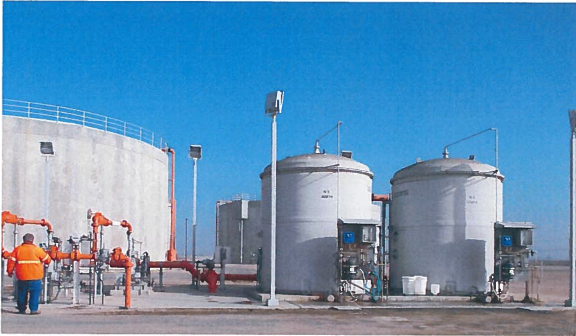
Figure F- 3 Existing Industrial Biogas Cleanup Skid
