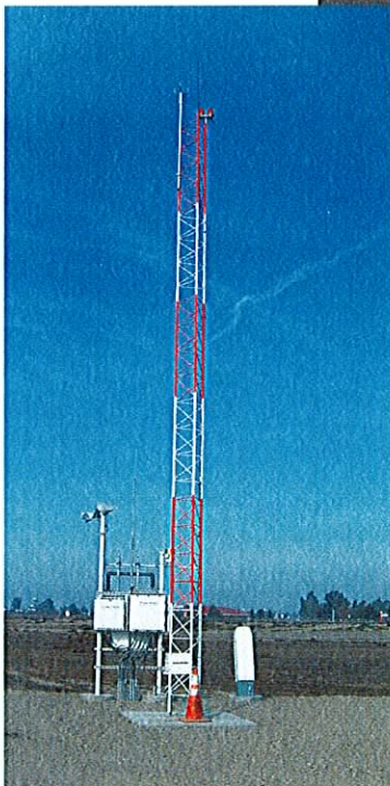
AWOS - Automated Weather Observation System
