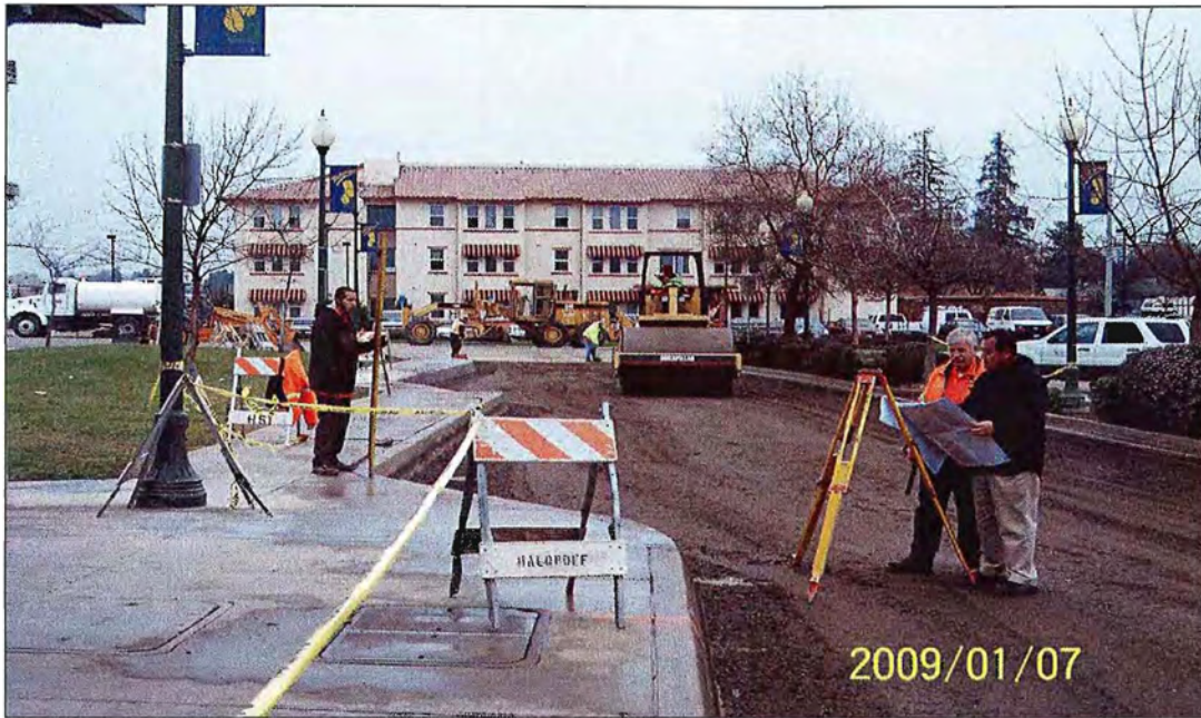
Engineering staff at work on a project to replace and strengthen the bus drive areas at the Transit Center.
