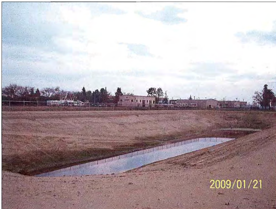
Working with the Redevelopment Agency to acquire underutilized property west of the railroad tracks, the Engineering Department oversaw the development of two new ponding basins along I Street just south of Cross Avenue. The new basins improve drainage in the downtown area to encourage new development.
