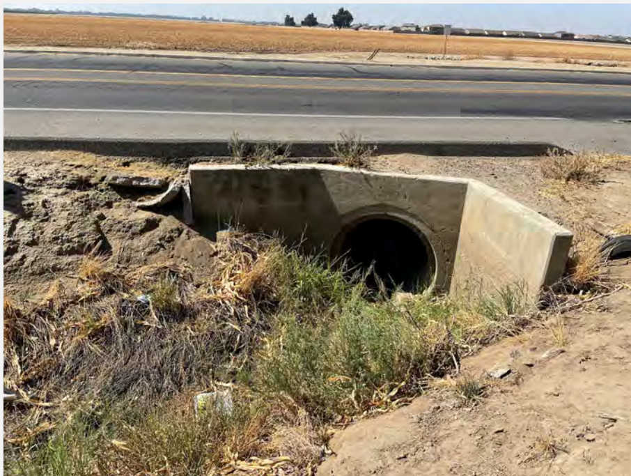
8. Bates Slough Ditch passing under East Bardsley Avenue on the southern subject property boundary.
