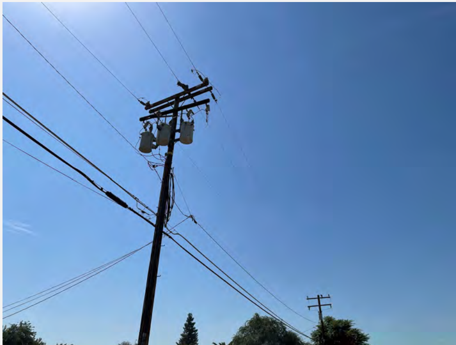
47. Pole-mounted transformers behind residences on Munson Road, along eastern subject property boundary.
