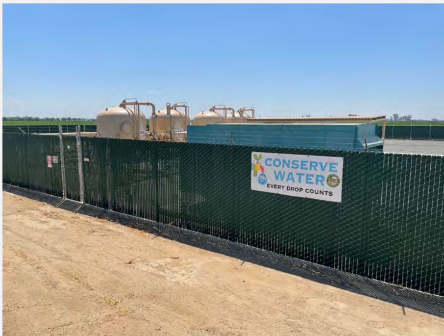
26. Municipal groundwater well and water treatment facility to the south of the subject property.
