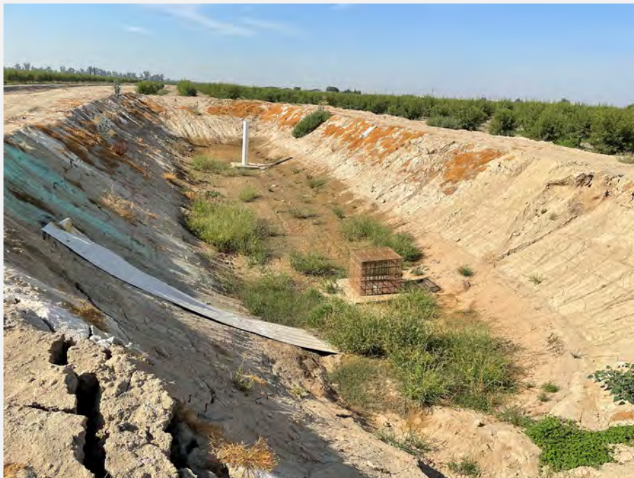
42. Storage pond located next to the irrigation supply groundwater wells, south of the filtration system.
