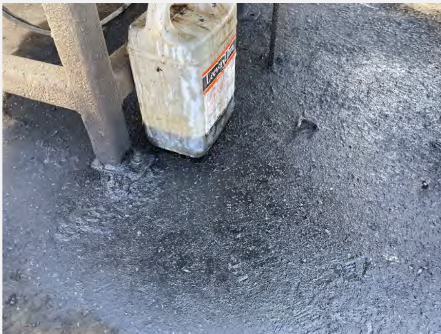
35. Oil staining/spill on concrete pad adjacent to irrigation supply well, and container of oil.
