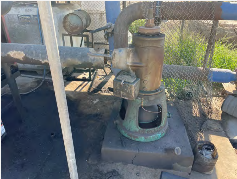
39. Diesel motor powered pump atop second irrigation supply groundwater well. Oil staining on concrete surrounding this well did not appear de minimis.
