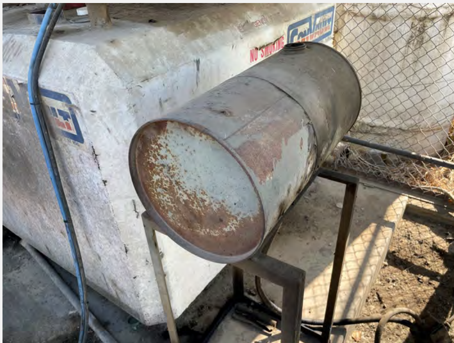
33. Hydraulic Oil storage tank located adjacent to diesel AST. Estimated to be approximately 50 gallons.
