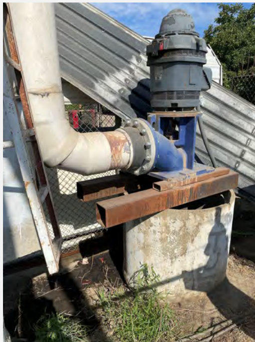
38. Electric pump atop one of the irrigation supply groundwater wells. Surface casing is approximately 3 feet. Interior casing/pipe is 12-inch-diameter iron pipe.
