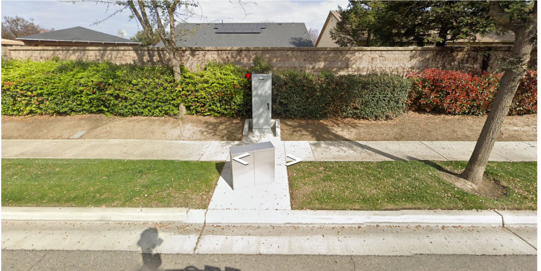
4. Morrison and Windmill Ave – Pole with Photo Cell
