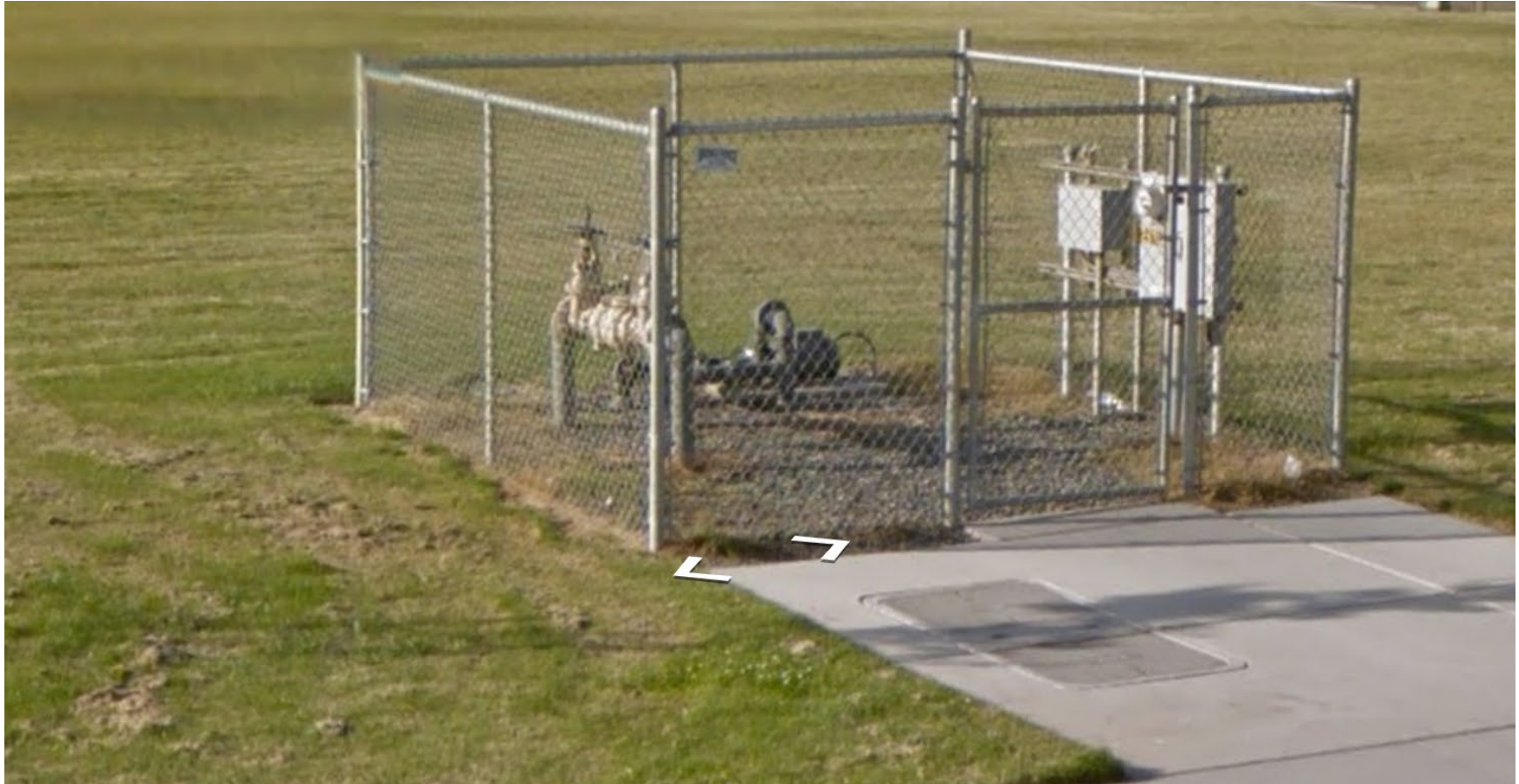
5. Sunrise Park – Lift station? – Pole with Photo Cell
