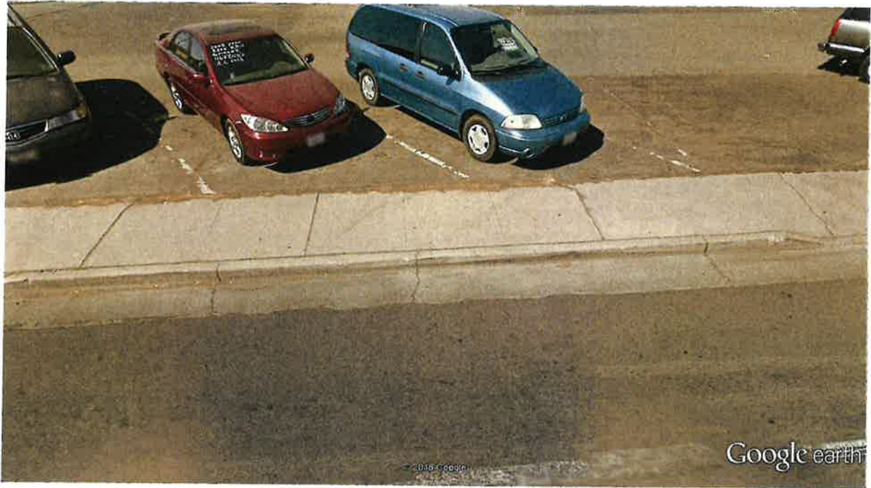
West Street – West side south of driveway approach at north end of project site. Major cracking in curb and gutter and moderate cracking in expansion joints of sidewalk.
