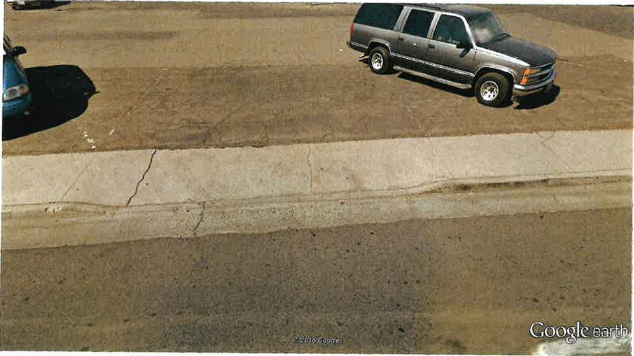
West Street – Driveway approach at north end of project site. Major cracking in curb and gutter and driveway approach. No accessible path of travel behind driveway approach.
