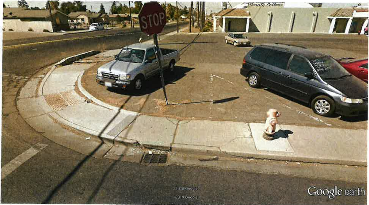
West Street – West side at curb return of Inyo Avenue. Severe cracking in curb and gutter, moderate cracking in sidewalk.
